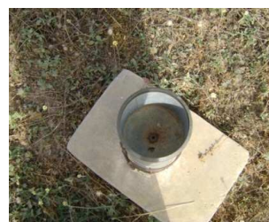
Fig. 5. Tipping bucket rain gauge.
